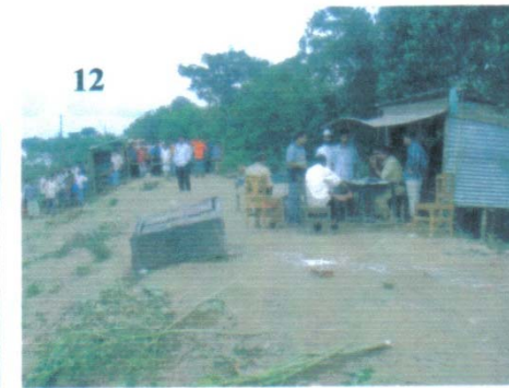
Photo(12) showing BWDB and security personals at the breach location
