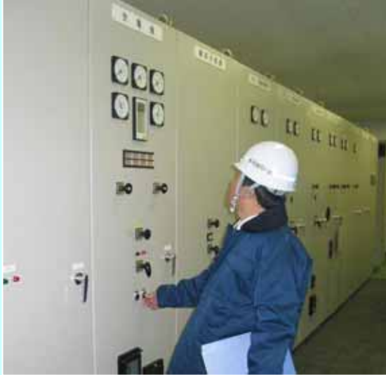
Power Supply Equipment inspection
