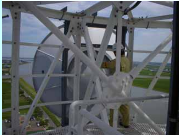
Communication Equipment inspection
