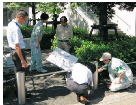
Installation practice for central disaster emergency communications network equipment (Headquarters)
