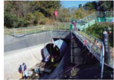
Bracing for an possible major earthquake (Inserting a steel pipe into the existing siphon) (Toyogawa Canal)
