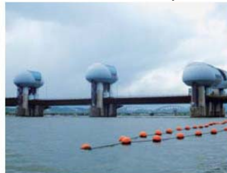
The gate at the Nagaragawa Estuary Barrage is widely opened to discharge flood water
