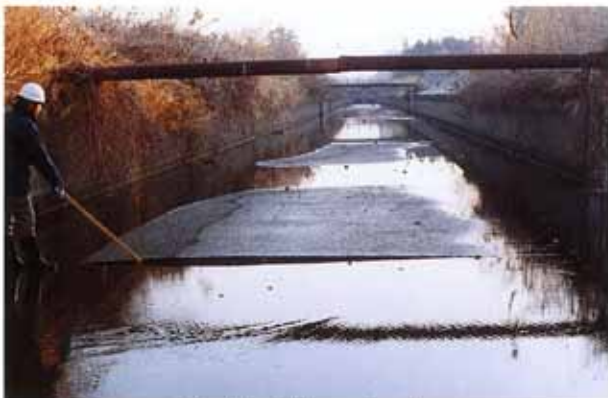
Lift of bed slab and cracks
