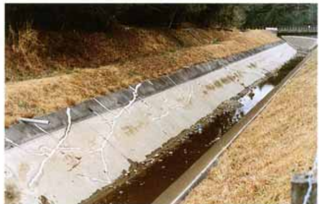
Cracks on concrete lining
