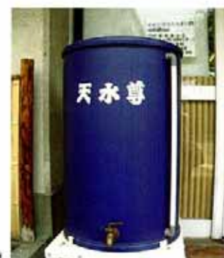
rain water barrel in Sumida Ward
