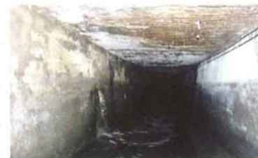
Deteriorated sewer pipe
