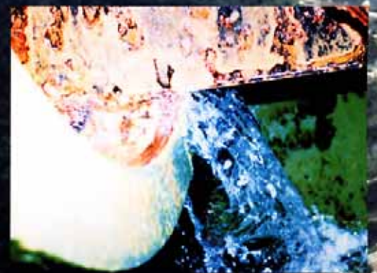
Aging and falling outlet facility
