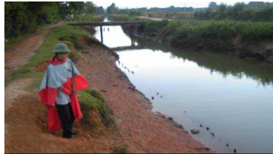
Photo: the eroded bank of irrigation canal
