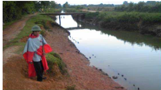
Photo: the eroded bank of irrigation canal
